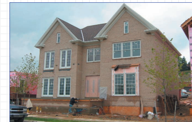
With the Icynene® application, this 7,700 sq. ft. custom home exceeded the SummerSet community's energy performance standards, resulting in initial savings of HVAC equipment costs and ongoing savings of utility costs.
