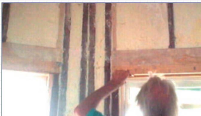
Icynene® is sprayed directly into the wall cavity. The foam softly expands to fill all of the cracks and crevices around the studs and window casings. Any excess foam is easily trimmed in preparation for drywall.
