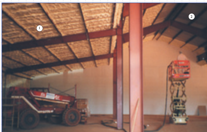
Icynene® applied directly to the roof deck. (1) Icynene® sprayed side, (2) unsprayed side.
